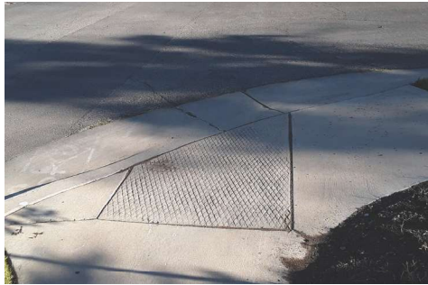
Figure 5: Substandard pedestrian ramps are prevalent along 900 E
